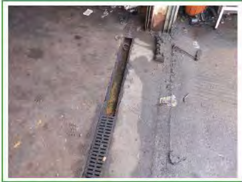
Photo No.72: Hydrocarbon staining and chemical presence noted in interceptor of Unit No.16 (hydrocarbon smell noted)
