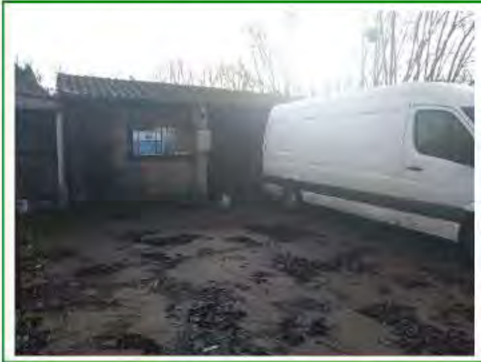
Photo No.52: Facing SE showing the frontage (northern) face of Unit No.20, located in a small-compound (PACM roofing)
