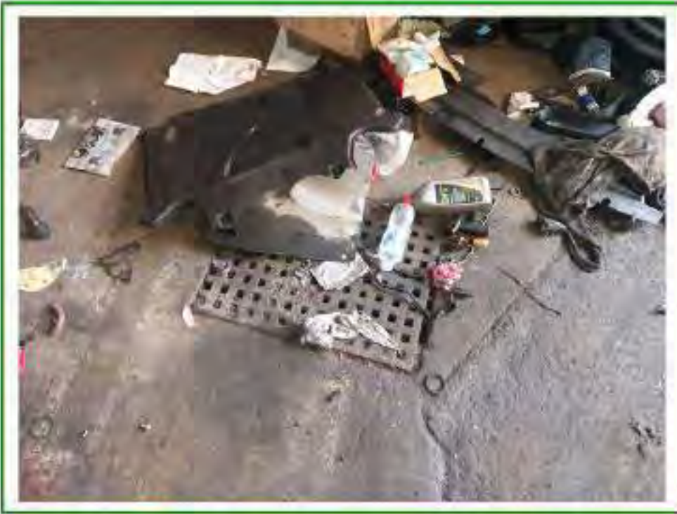
Photo No.70: Open drains – likely associated with former mill usages – noted within Unit No.16 (at least 2 No. noted here)
