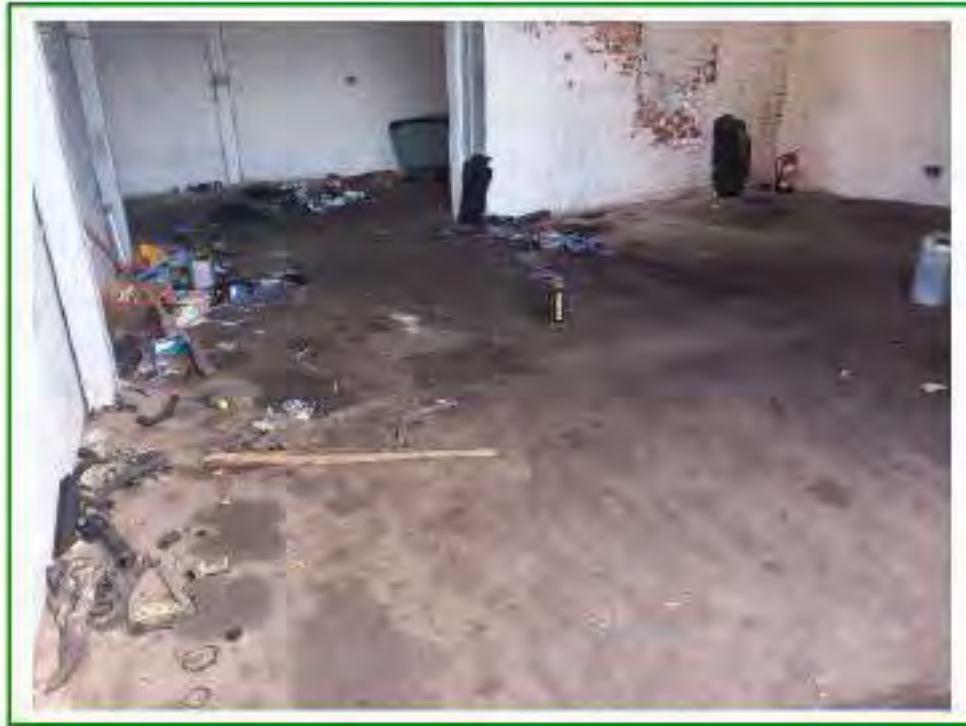
Photo No.68: Interior of Unit No.16 showing scattered debris and significant hydrocarbon staining on flooring
